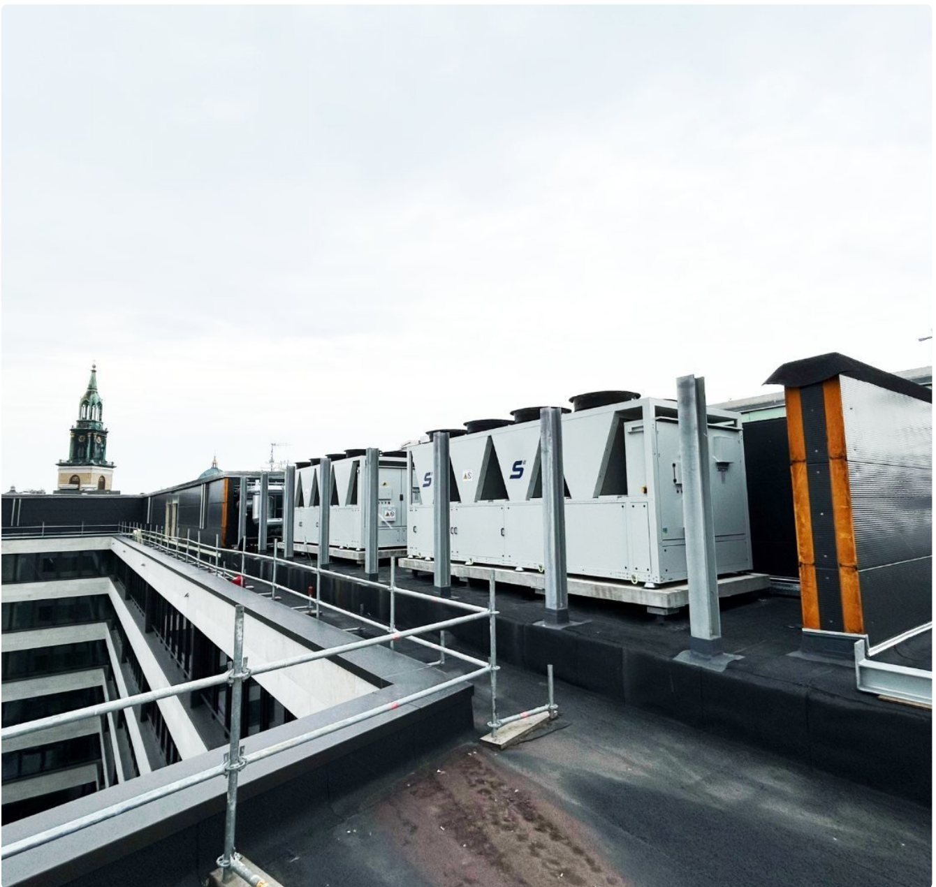
Secon's STRATOS VP series propane chillers installed on the roof of the C1 office building in Berlin. Photo credit: Secon
