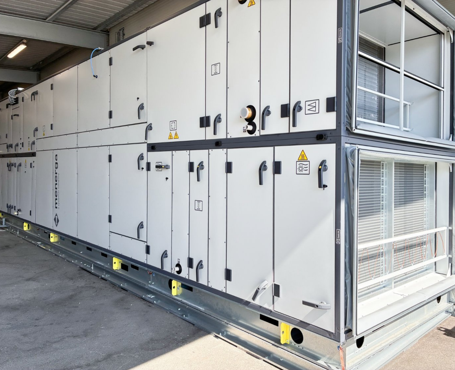
A Menerga CO 2 mpass at the Maribor factory in Slovenia. Photo credit: Systemair
