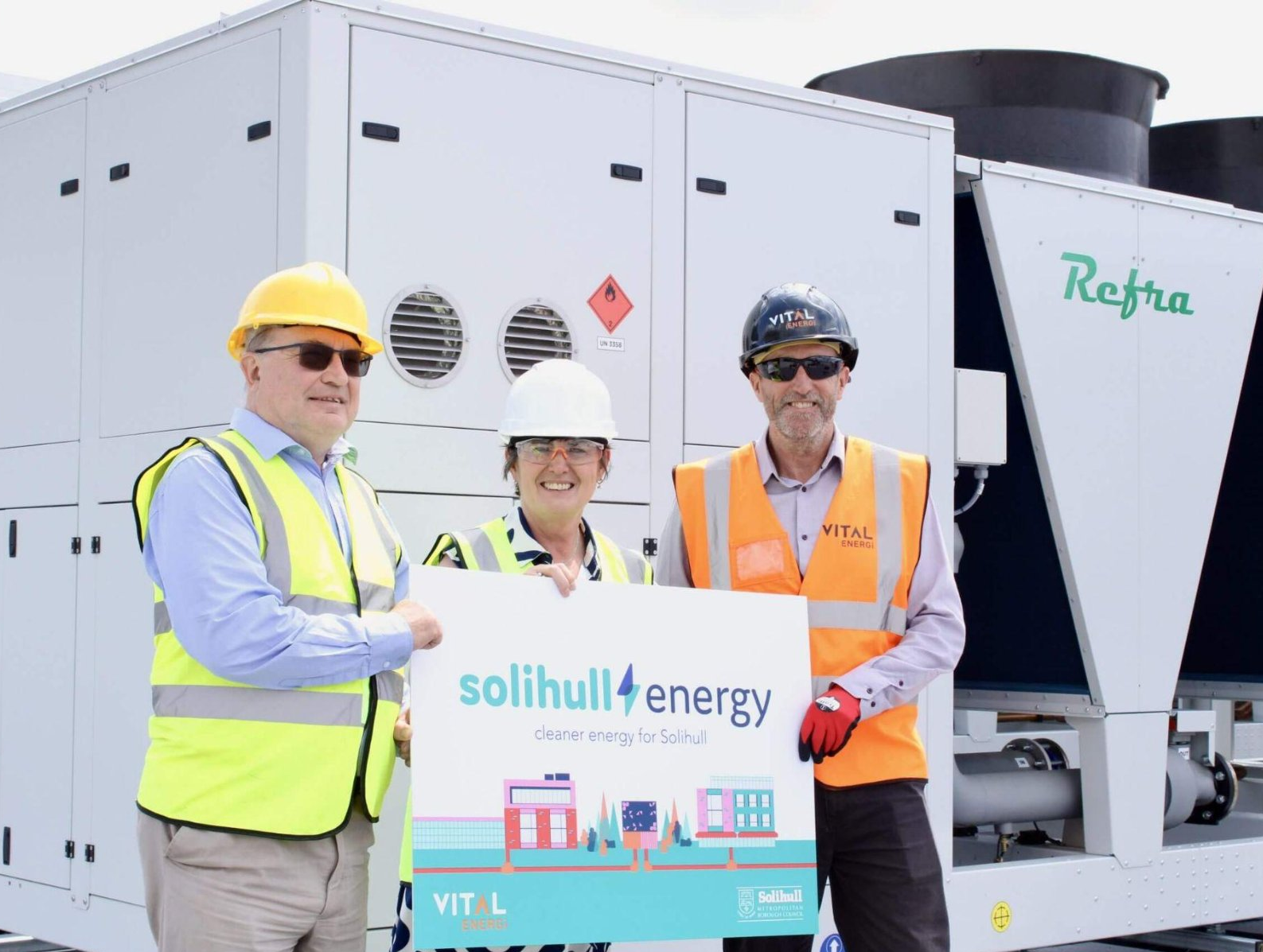
Refra's propane heat pumps installed at the Solihull district energy network. Photo credit: 2025 Solihull Metropolitan Borough Council
