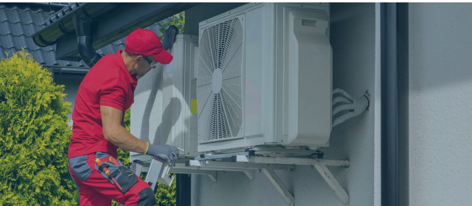
Image. HVAC technician installing or servicing an outdoor air conditioning unit on a residential building. (Source: Shutterstock)
