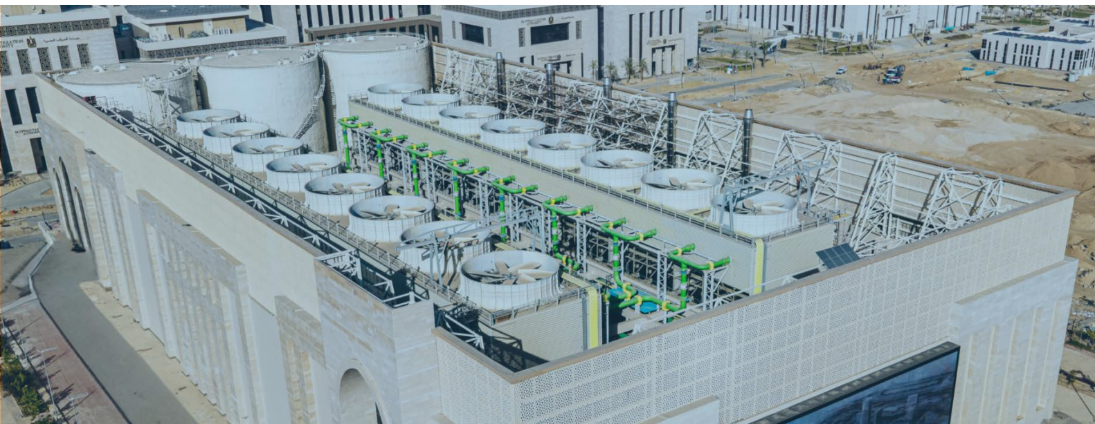
Image. A district cooling plant in Egypt's New Administrative Capital, near Cairo City.
