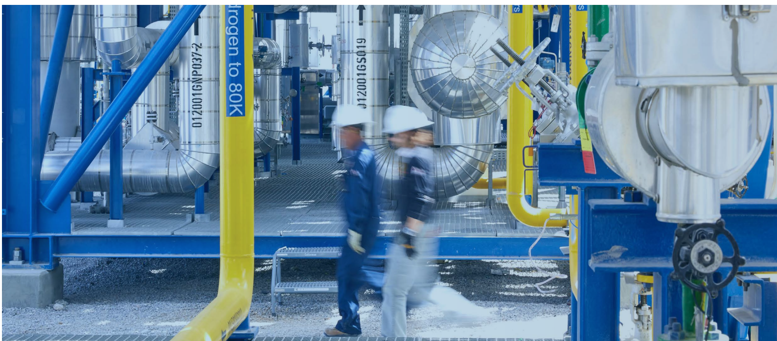
Image. Air Liquide liquid hydrogen production facility. (Source: Mediakit)
