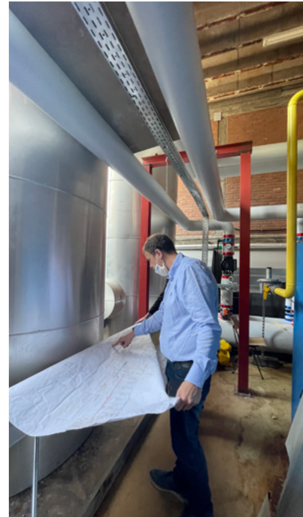
District heating network at Kortrijk Weide, Belgium ©Agata Smok
