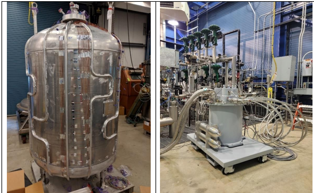
Figure 1. CryoFILL tank & BAC tubes (left). Cryocooler cold head enclosure (right).
